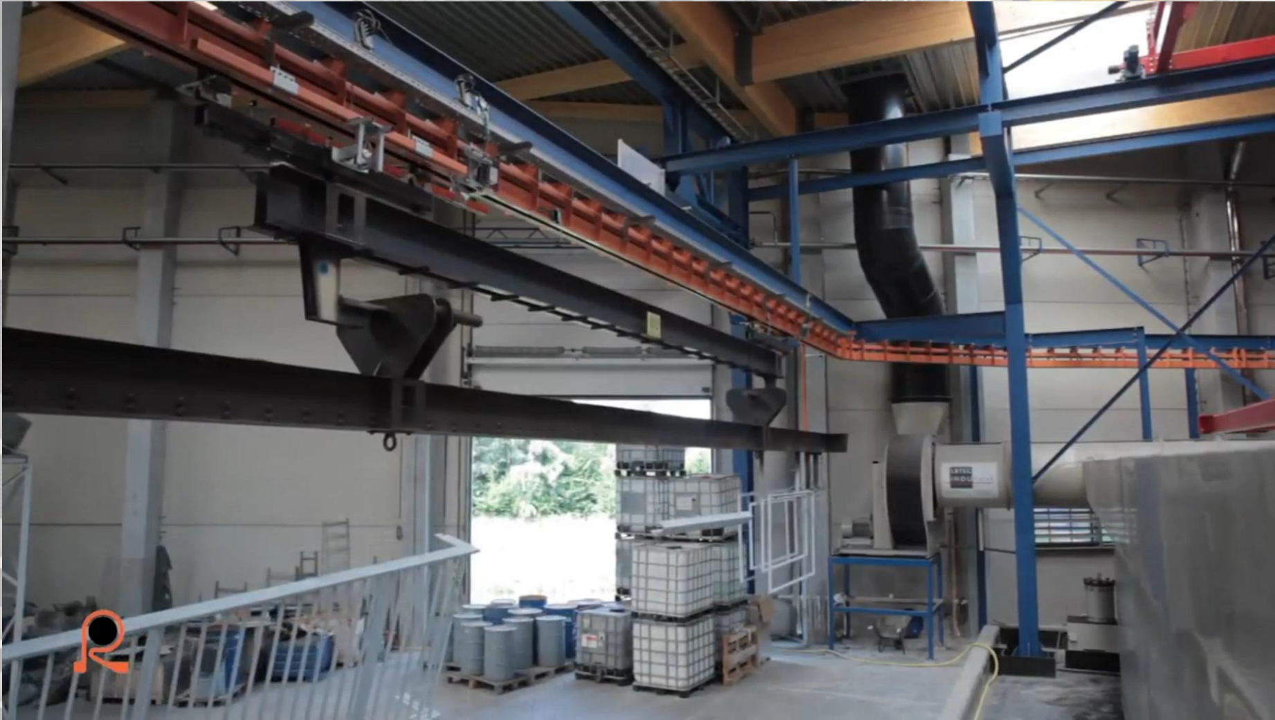
Transfer Of Flight Bar From P&F Conveyor To Dip Pre-Treatment Crane
